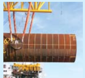
All 140 turbine foundation monopiles were installed using the first set of lifting slings. After completion Lloyd's proof loaded the slings and recertified them for continued use.
