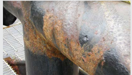
All rope contact surfaces need to be smooth and free of rust, corrosion, metal burrs, and sharp cutting edges.
